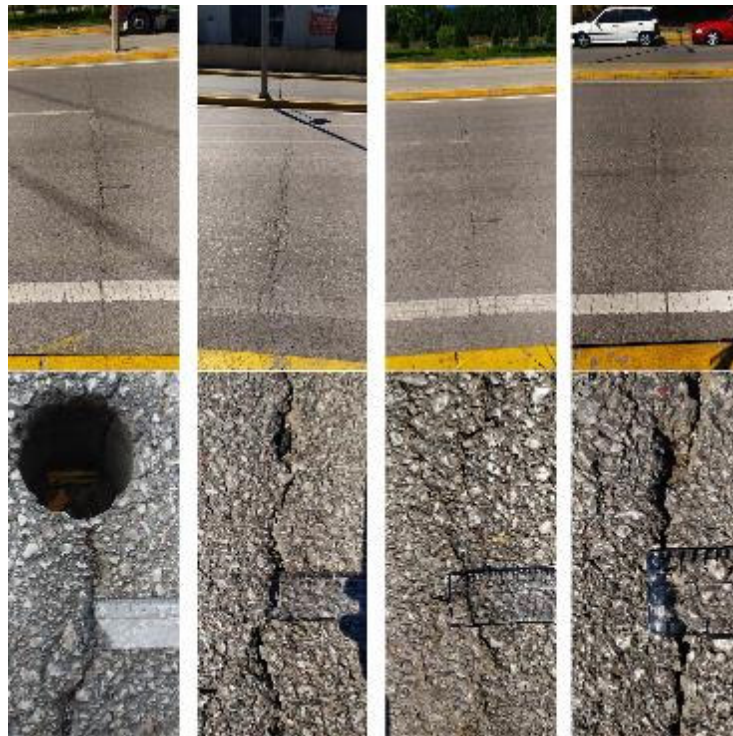
Figure 8. In situ examination of reflection cracks (2022)
